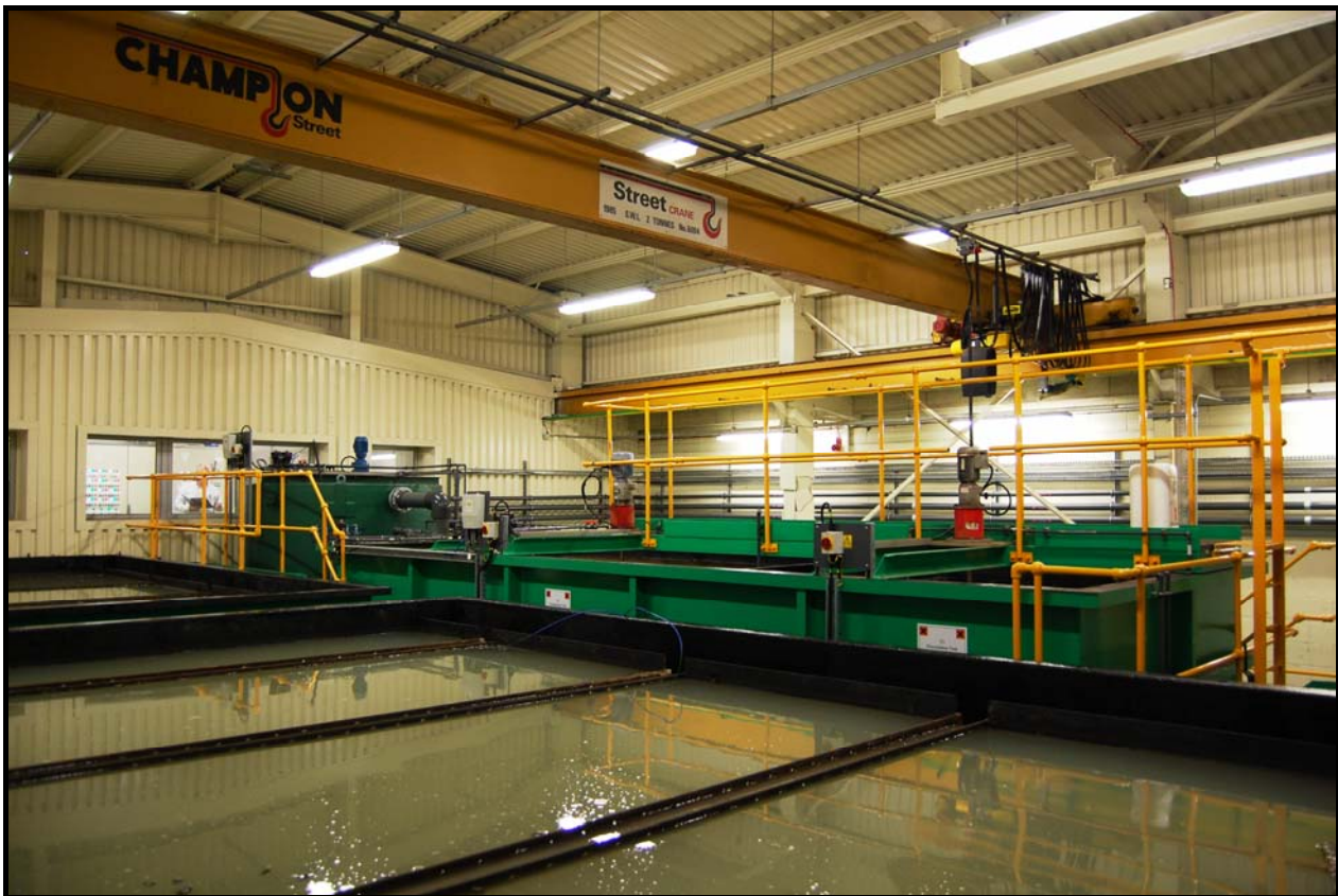
Treatment and Settlement Tanks
