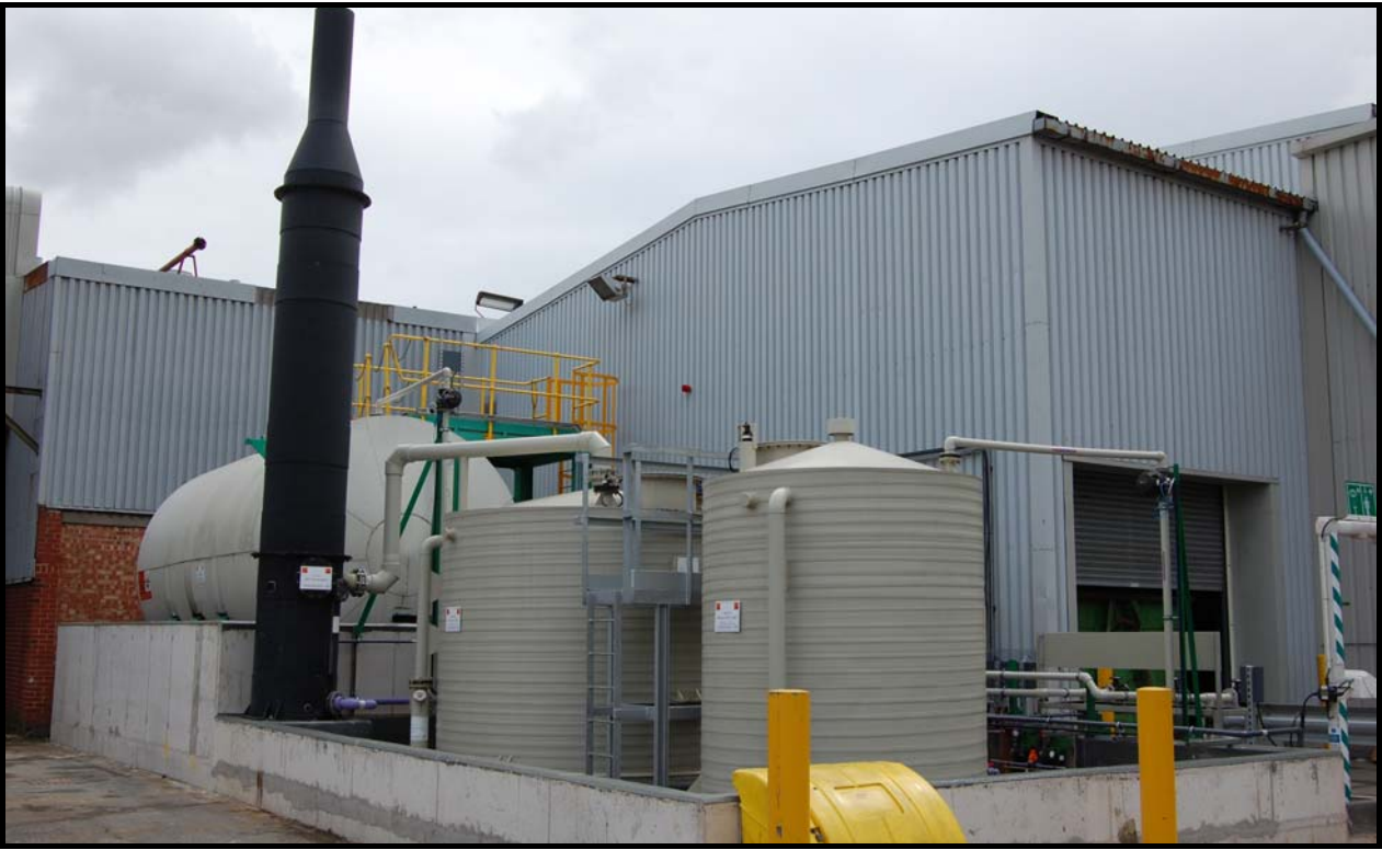
Bulk Chemical Storage Tanks
