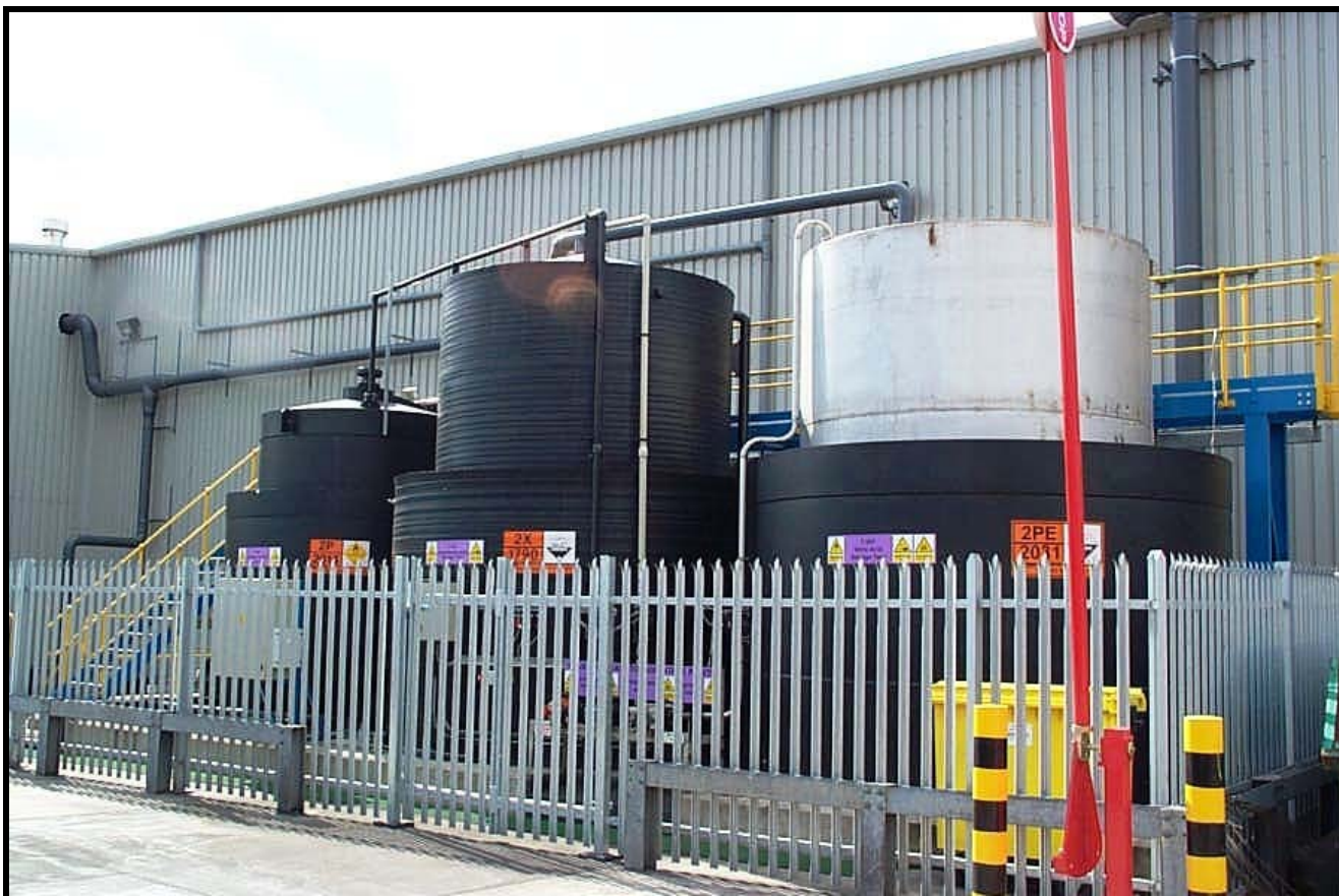
Bulk Pickling Chemicals Storage Facility
