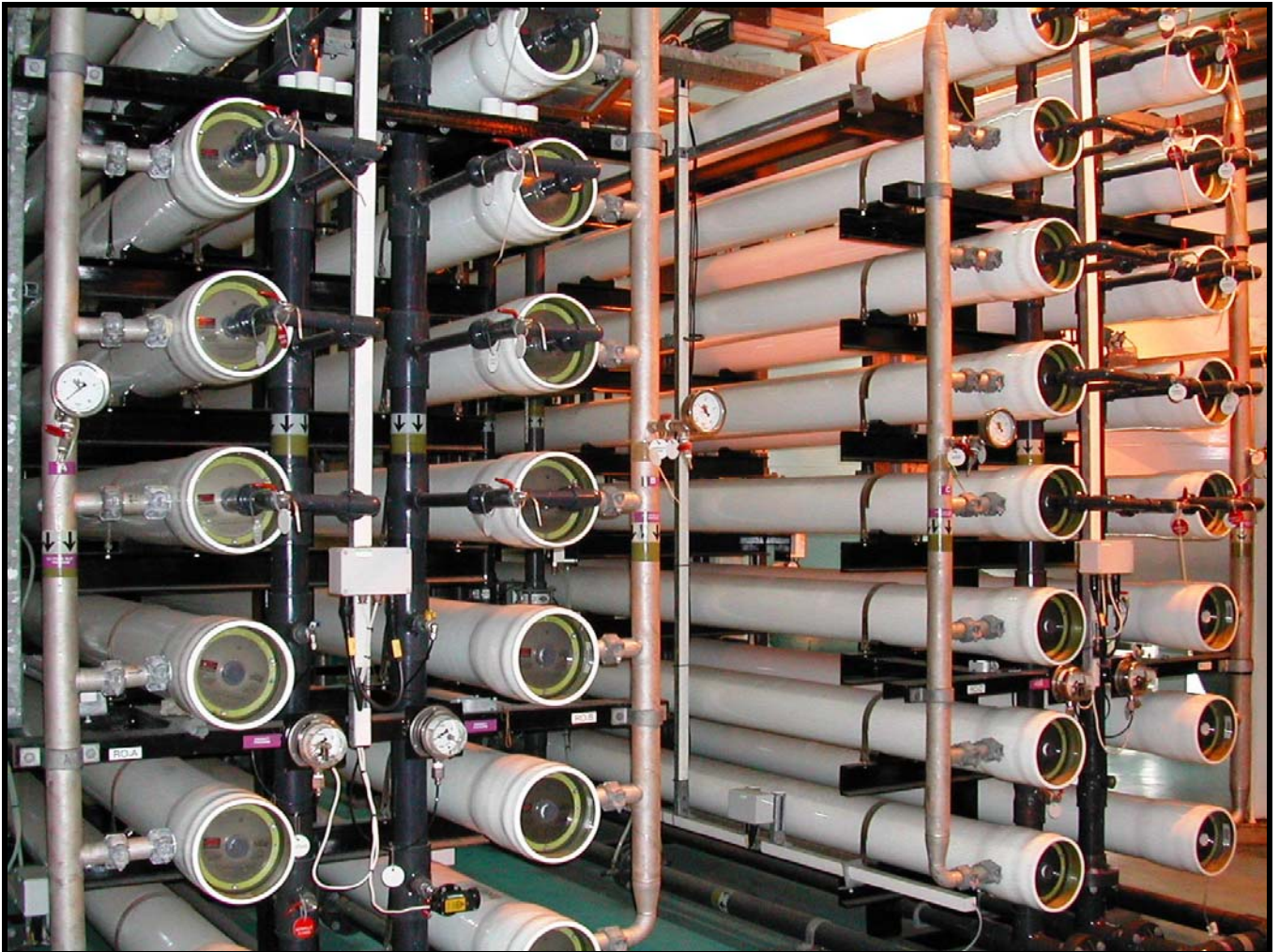
Primary Reverse Osmosis Units
