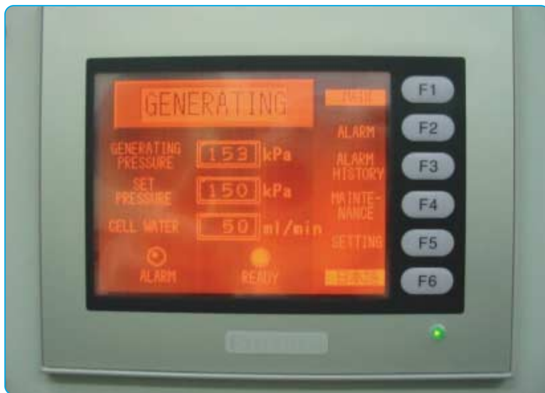
H-300 Unit in "Generating" Mode
